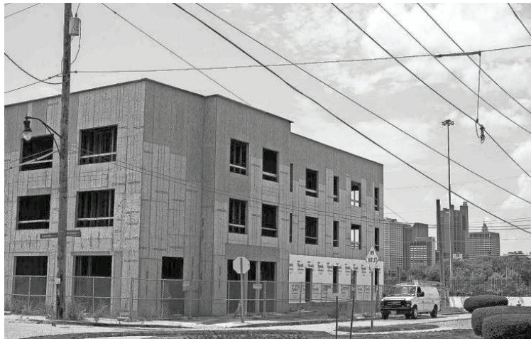
Construction is underway at the Shiloh Apartments at Hamilton and Mount Vernon avenues in the King-Lincoln-Bronzeville District. The project includes 82 apartments. COURTNEY HERGESHEIMER/COLUMBUS DISPATCH
